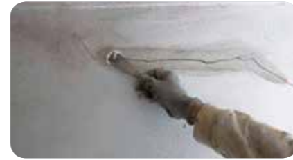
STEP 3: Apply the lightweight acrylic putty STATUS ONE COVER , with a spatula, over the crack opening.
