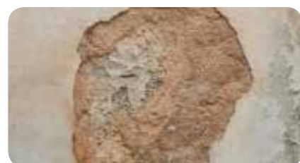
Due to aging, parts of plaster become loose and finally detach.
