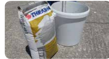
STEP 5: Leveling of surface with a spatula, removing the material in excess.
