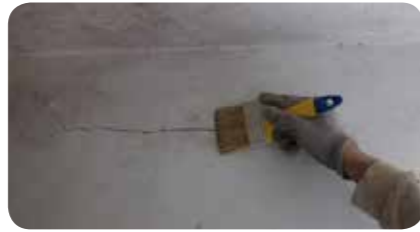
STEP 2: Clean thoroughly the crack opening, with a brush, from dust and loose particles.
