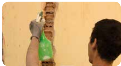
STEP 1: Clean thoroughly the surface of application from dust and loose particles, irregularities, etc. Then, spray water on the surface.
