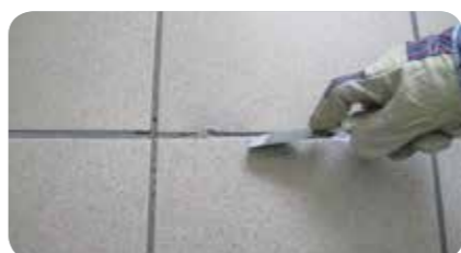
STEP 1: With a metal spatula remove the loose particles of the problematic tile grout.
