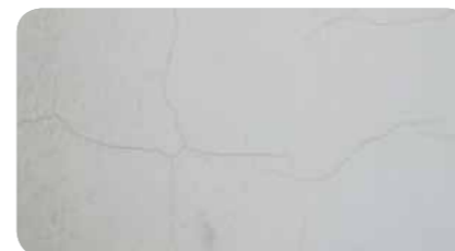
There are cases of small hair cracks existing on the surface of plaster. They should be covered with a product be flexible enough to withstand thermal expansions, protecting our masonry.
