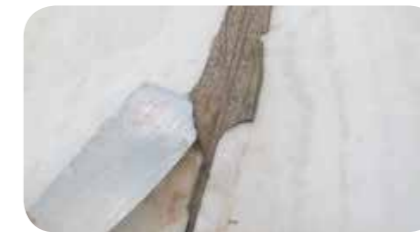
STEP 1: Clean the surface of the joint thoroughly, by removing the existing sealant with a metal spatula at the entire length and width of the joint.
