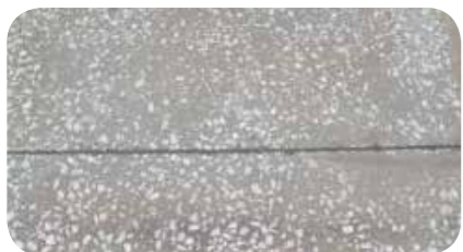
If a joint is problematic, it needs waterproofing to avoid humidity problems.
