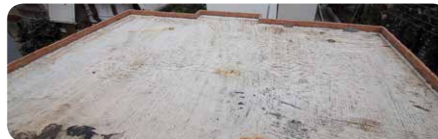
For common substrates, apply FLX 380 ROOF SEALER . It has high elasticity and is suitable for surfaces in severe contraction and vibration. Once we make the necessary repairs explained in the previous steps, we proceed with the preparation of the substrate.
