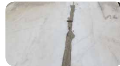
Marble application at parapets is used for giving a luxurious style at the construction. After some years, the sealing material maybe damaged. In this case it needs to be replaced in order to prevent the inflow of humidity beneath the marble.
