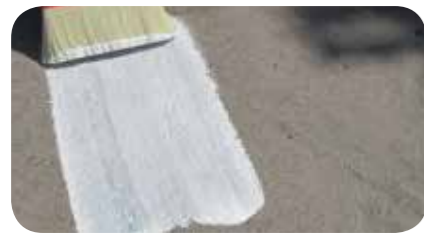
STEP 3: Once the primer has dried, apply the first layer of acrylic, fiber-reinforced, waterproofing brushable membrane, FLX 382 PLUS .
