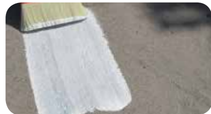
STEP 6: After the first layer of FLX 382 PLUS has dried, a second layer is applied along the crack.
